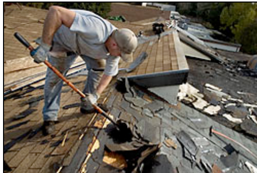
Skyles Morgan tears up a roof Monday at a Davis duplex. His employer, the roofing company Carder & Daughters, uses a voluntary federal program to check the citizenship status of potential employees. Congress is considering legislation that could make the program mandatory.
